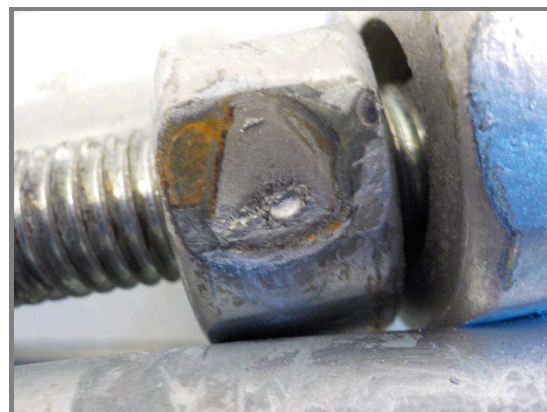
Fig.2 – close up of failed spot weld on nut showing reduced cross-sectional area of bonding
